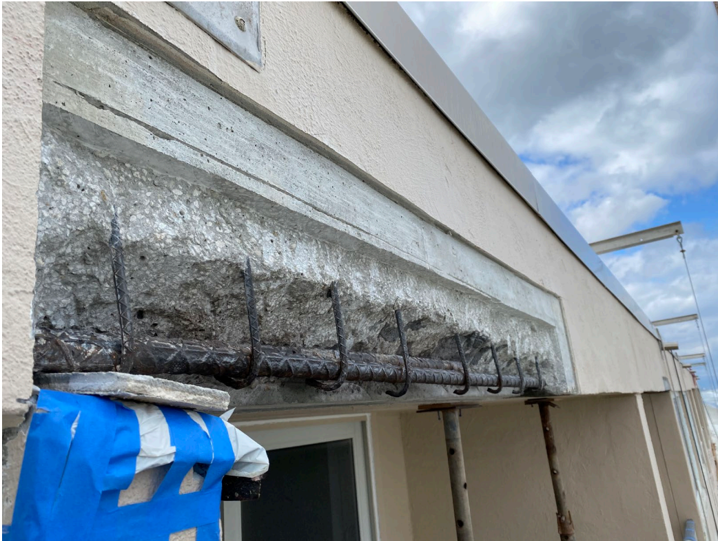
Picture 1: Spall edge on Unit 705
